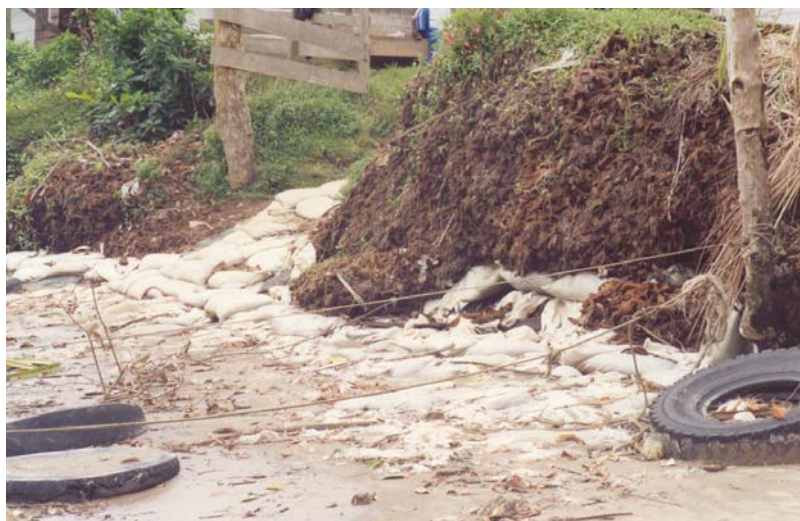
Picture 13: Campo beach with sand bags / tyres used bags / tyres used as protective structures against erosion
