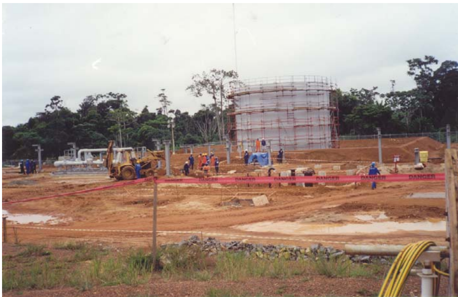
Picture 29 : Construction work at the Kribi terminal of the Cameroon-Chad pipe line project.
