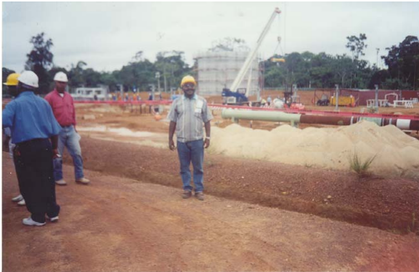
Picture 30 : Broad view of the Construction work at the Kribi terminal of the Cameroon-Chad pipe line project.
